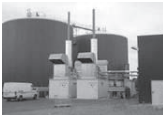
Picture 2. Dairy „Lazar“ - Blace - The first biogas power plant in Serbia
