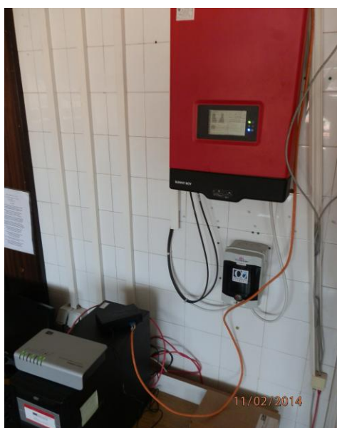
Figure 2. Part of the PV plant inside the Laboratory.
