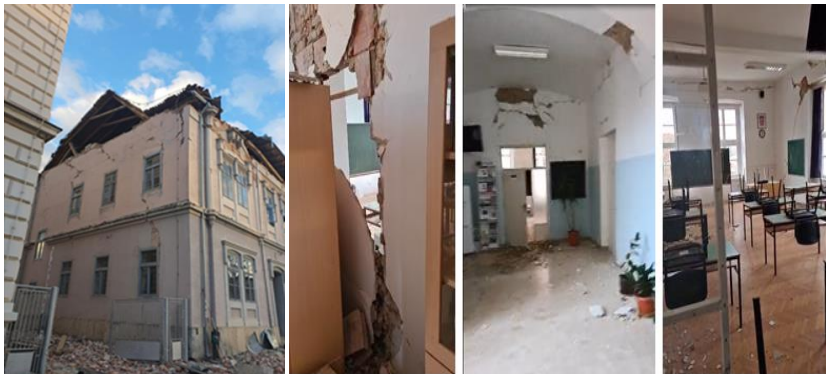
Figure 4. Damages in schools in Petrinja (source: Nenad Bijelić)
