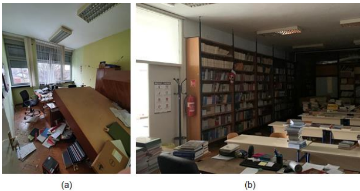
Figure 5. Comparisons of (a) inadequate and (b) sufficient anchorage of building content in 1962 university building (Učiteljski fakultet Petrinja) (source: Marko Bartolac)
