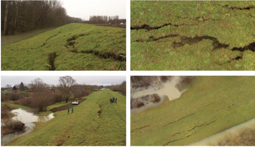
Figure 6. Embankment / levee failure by river Sava in Galdovo (source: Croatian Waters Archive)
