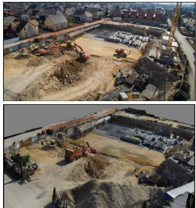
Figure 10: Realistic photography of construction site (upper); 3D model generated from aerial photos using the UAV (lower)
