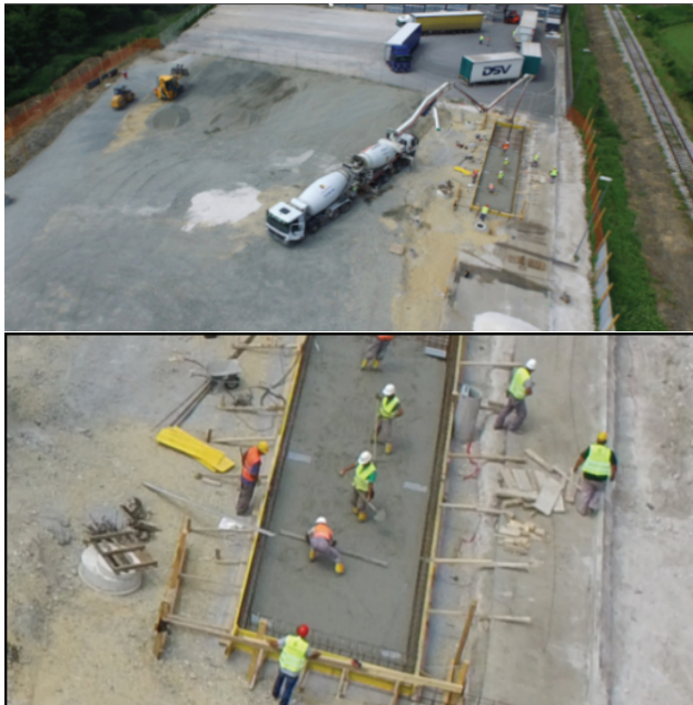
Figure 7: Aerial photograph of the construction site (upper); Magnified picture to monitor the use of protective equipment (lower)
