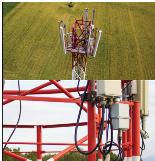
Figure 8: Examination of construction of the base station (upper); Detailed view of the construction (lower)
