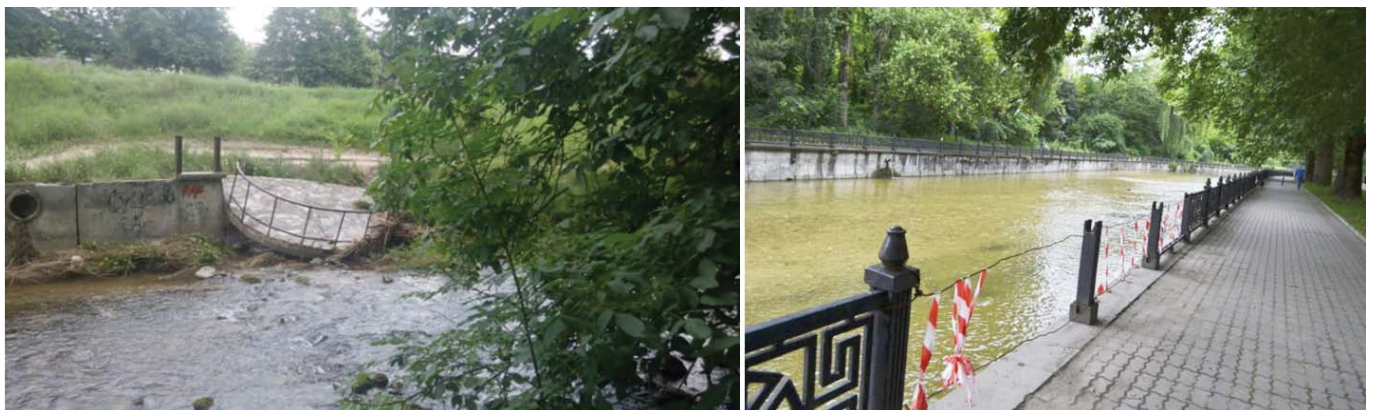
Figure 1: The embankment of the river. Salgirin Simferopol City requires repair and reconstruction
