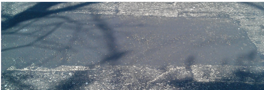
Figure 1: Section of the newly repaired pavement by cold milling in the Khabarovsk Krai
