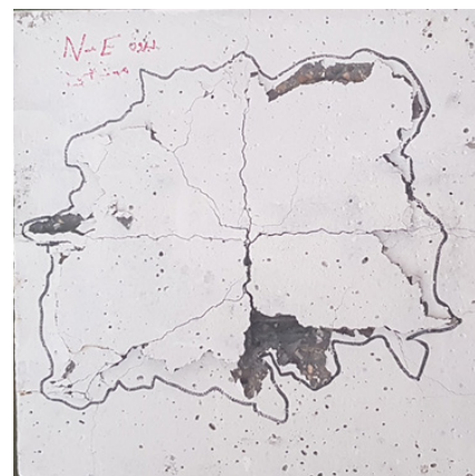
Figure 17: Failure pattern of NW-28
