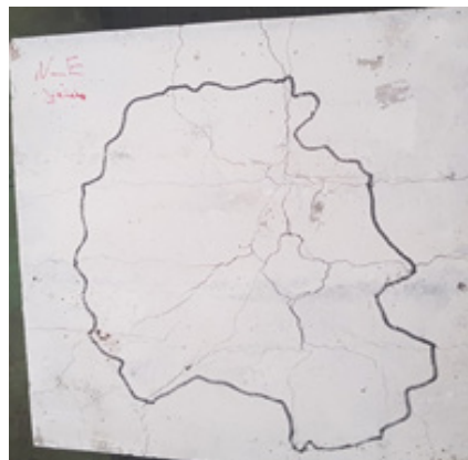
Figure 10: Failure pattern of HH-28
