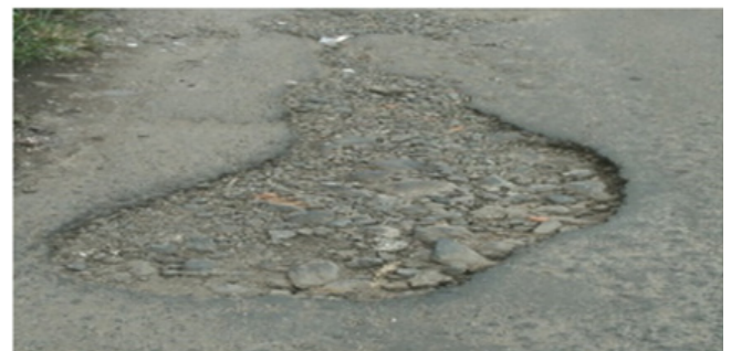
Figure 3: Damage to Rd Ciherang and Rd Pemuda
