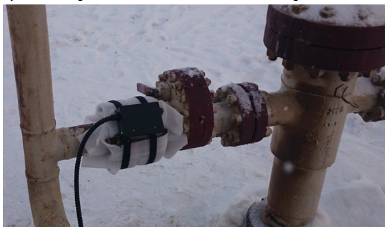
Fig. 2.2.2 - Working condition of INK-150
