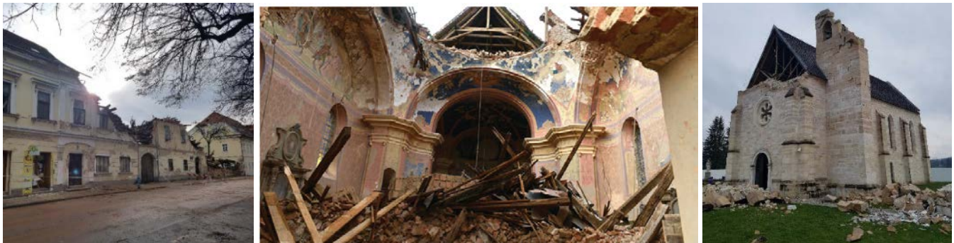
Fig. 4. Petrinja earthquake, (a) center of Petrinja [14], (b) Church of St. Nikola and Vid, Žažina (source: Ministry of Culture and Media) (c) Church Mother of God, Gora [14]
