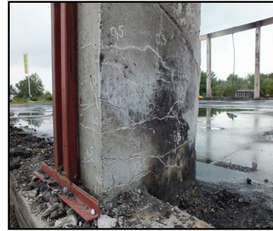
Figure 5: Horizontal cracks due to flexion of column (during the collapse of roof structure)
