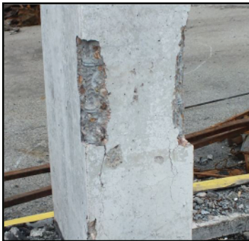
Figure 3: Cracking, separation and peeling of concrete along the column edges (up to the main longitudinal reinforcement), pronounced change in aggregate colour, net-like fissures
