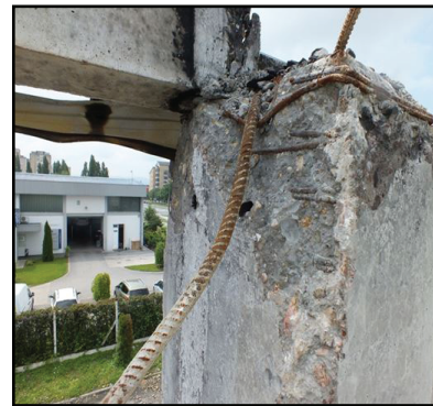
Figure 6: Crumbling of concrete in the supporting zone, peeling of surface and protective concrete layers, deformed stirrups and anchors, change in aggregate colour
