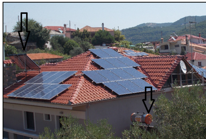
Figure 4: Wrong orientation PV panels
