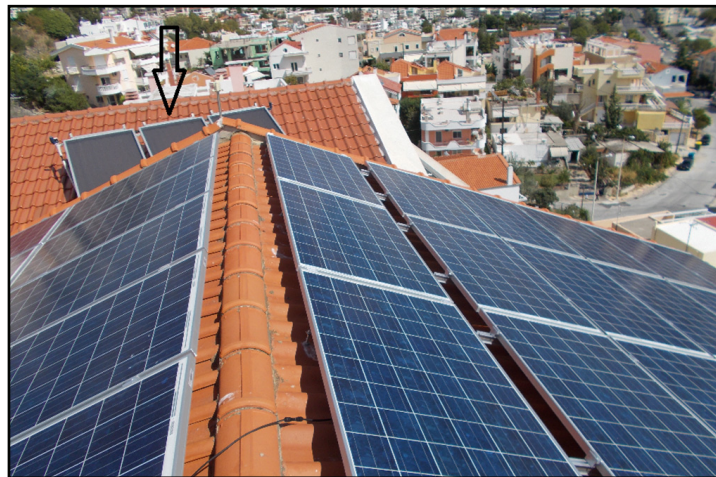
Figure 5: Panels oriented east-west direction
