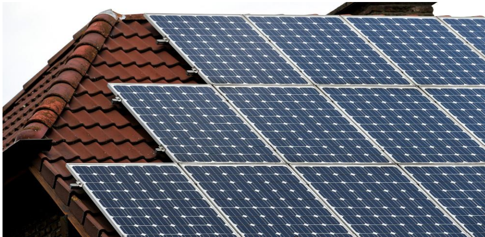
Picture 2. Installed solar panels on the roof of the building
