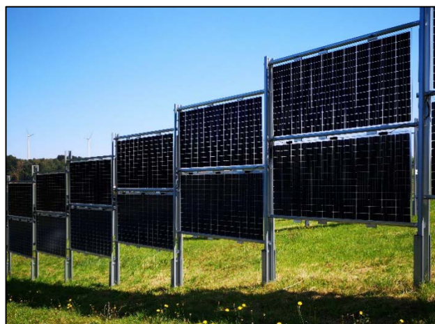
Fig. 1. Mounting system with vertically erected bifacial photovoltaic modules.
