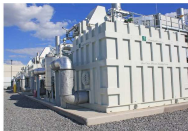
Commercial FC Power plant in Germany
