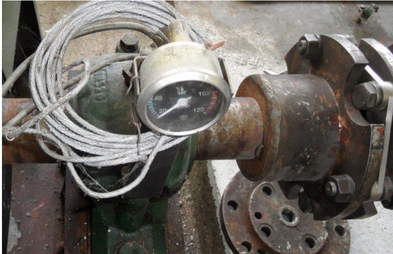
Figure 2 – Damage to the flange of flexible elastic couplings on the flywheel shaft of a mini hydro power plant
