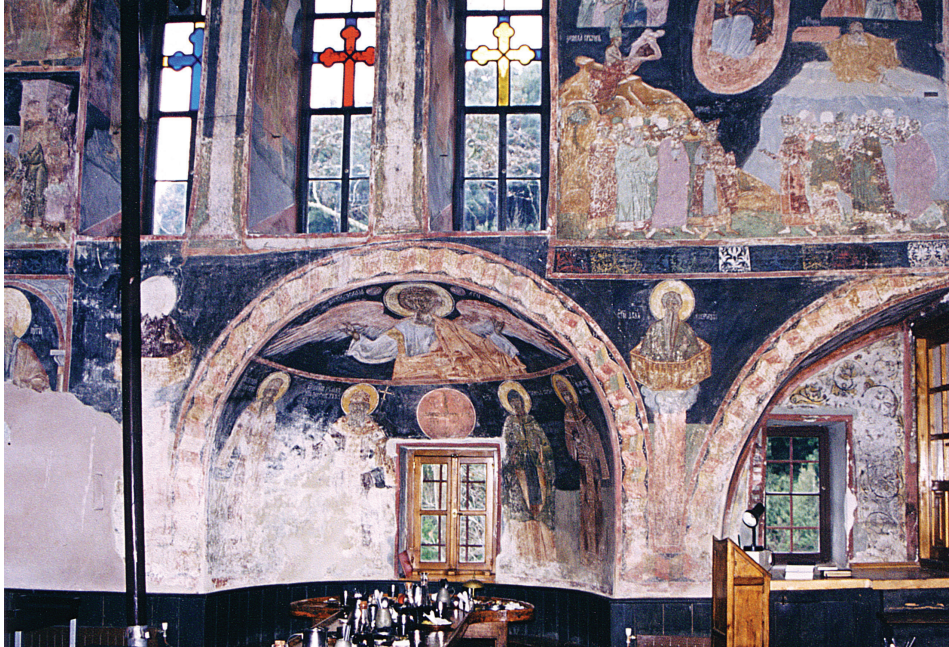
Fig. 2. Hilandar refectory, view of the south wall with the apse (photo by Nikolaos L. Dionysopoulos)
